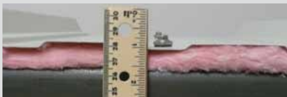
Teks Stand-Off with Scots Head Style (5/8" Stand-Off) (26 ga. panel, 17 ga. girt, 6" fiberglass insulation)
